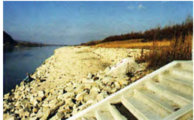
Figure 2. Gravel-bank inshore structure under construction with two ripraps. Nowadays, after filling of the impoundment, only parts of the upper riprap are visible (Waidbacher).
