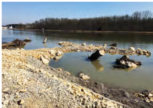
Figure 1. Installed 'eco-berm' at Offingen hydropower plant. On the opposite side there is still the traditional concrete embankment.
